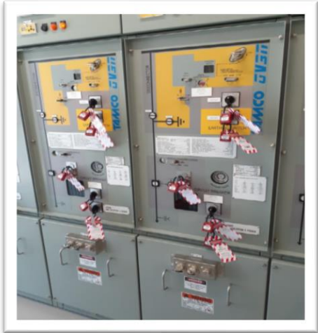
Safety testing and tagging of equipment in the substation
